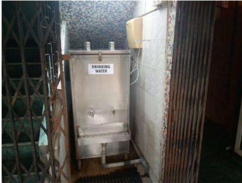
Drinking Water Facility with signage
