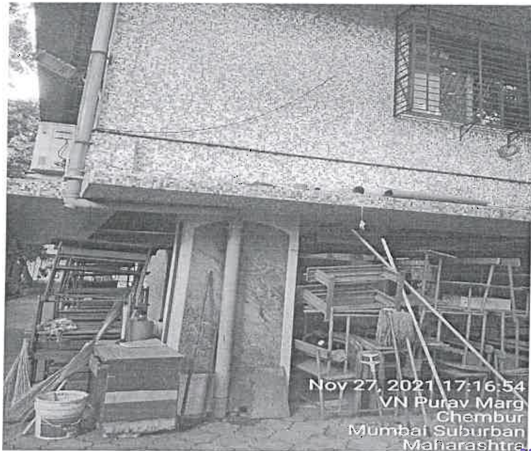
Rain Water Harvesting Discharge Point
